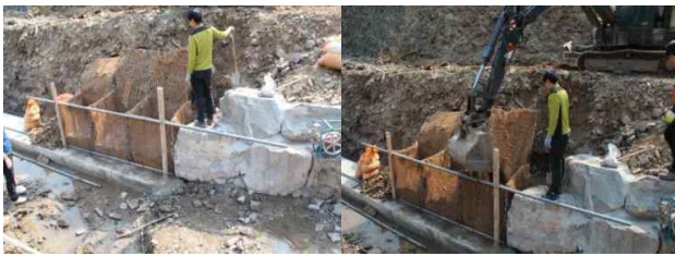
Keeping inside stone, forest soil, seed and vegetation base materials in revetment of using gabion systems
